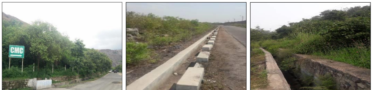
Garland drain in the area
