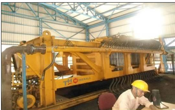
Mechanical tailings de-watering system
