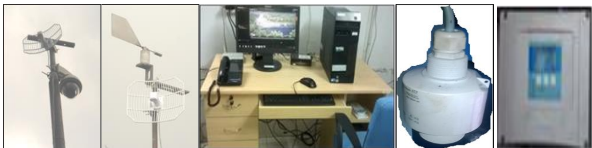
Zero Discharge Monitoring System installed at site (Power Plant)
