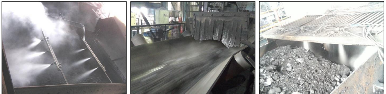
Dry fog dust suppression system in crushing units
