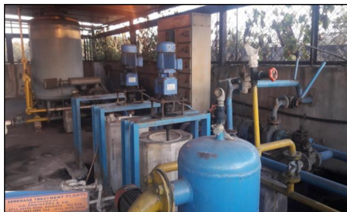
Sewage Treatment Plant (0.24 MLD) at West Bokaro
