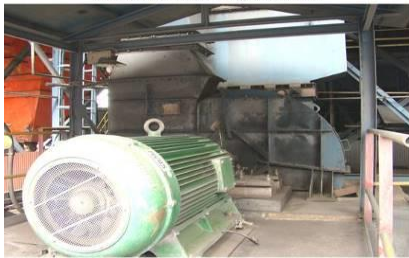
New FD Fan with Silencer leads to significant reduction in noise generation
