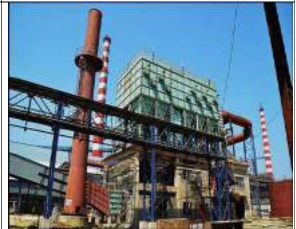
Stack: Bag Filters, ESP, Scrubbers & Cyclone
