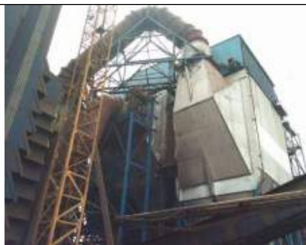
Sinter Plant 3 New Waste Gas ESP
