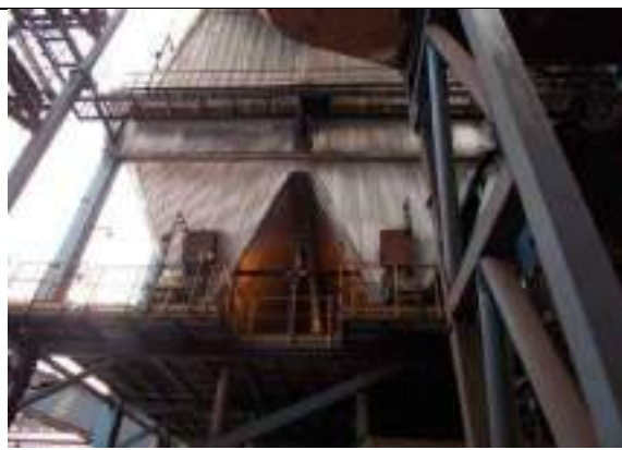
Sinter Plant 3 Refurbished ESP
