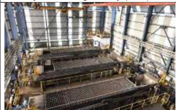
Blast Furnace Sludge Drying Plant
