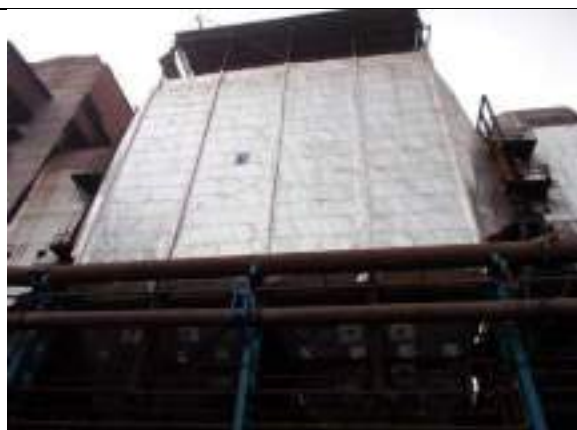
Sinter Plant 2 Waste Gas ESP
