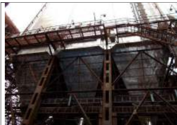
Sinter Plant 1 Waste Gas ESP
