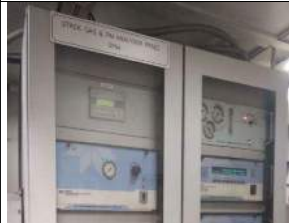
Stack Analyzers & Monitoring
