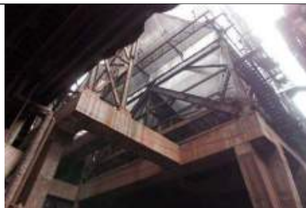
Sinter Plant 2 Refurbished ESP
