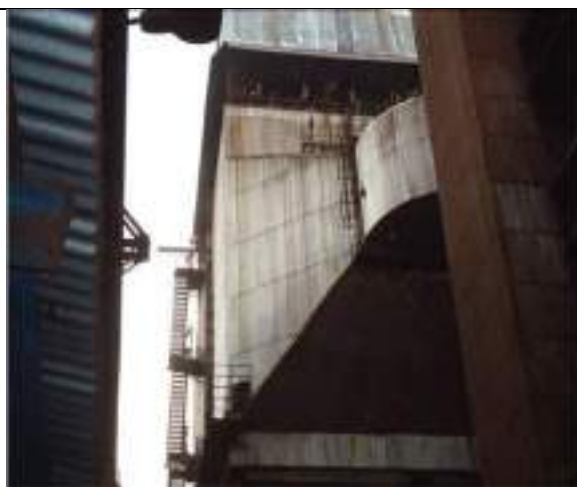
Sinter Plant 2 New Waste Gas ESP
