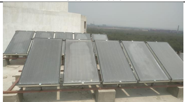
Solar panels installed above high rise buildings
