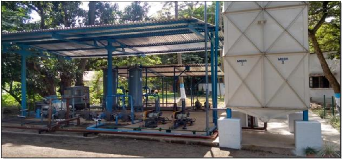
Sewage Treatment Plant Installed at FAP, Joda
