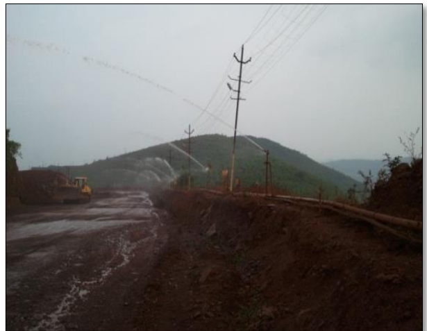
Stationary Water Sprinkler
