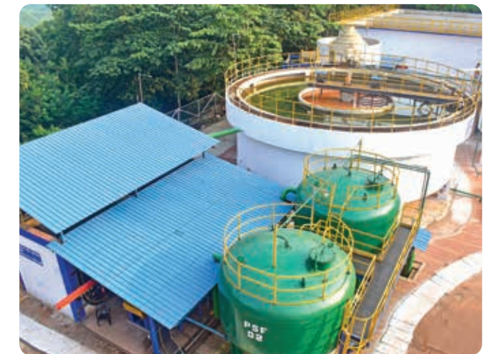
Water treatment plant at Noamundi, Jharkhand
