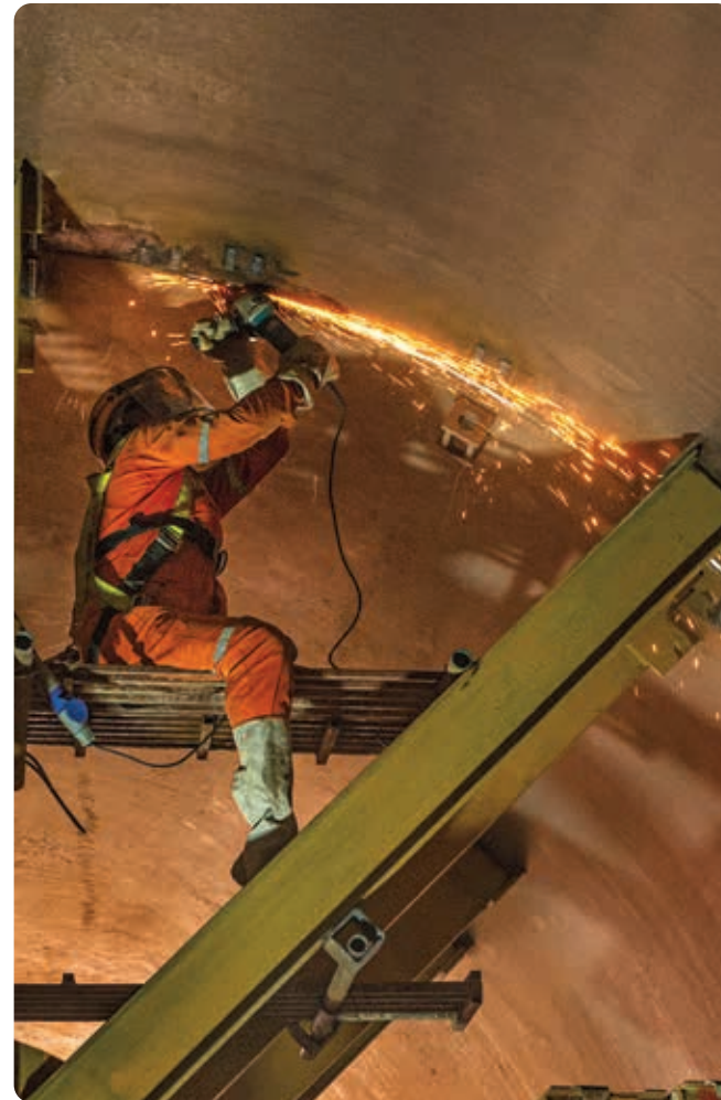
Blast Furnace, Tata Steel Kalinganagar Works
