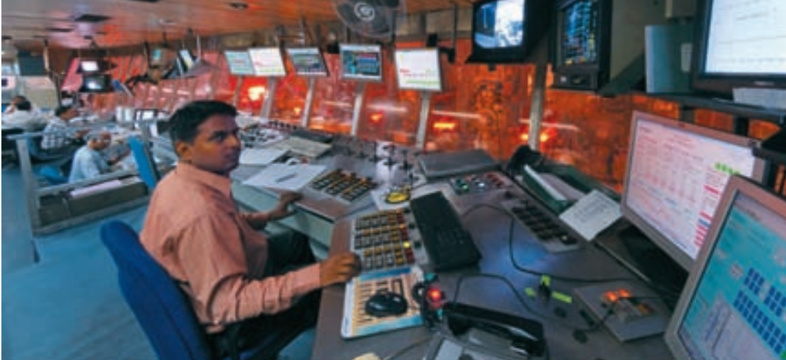
The state-of-the-art Hot Strip Mill control room at the Jamshedpur works.
