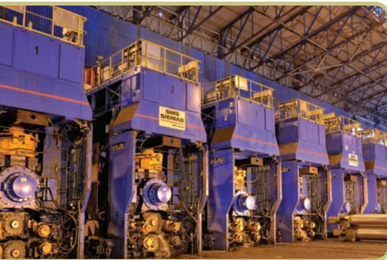
TSCR Facility at Jamshedpur Works
