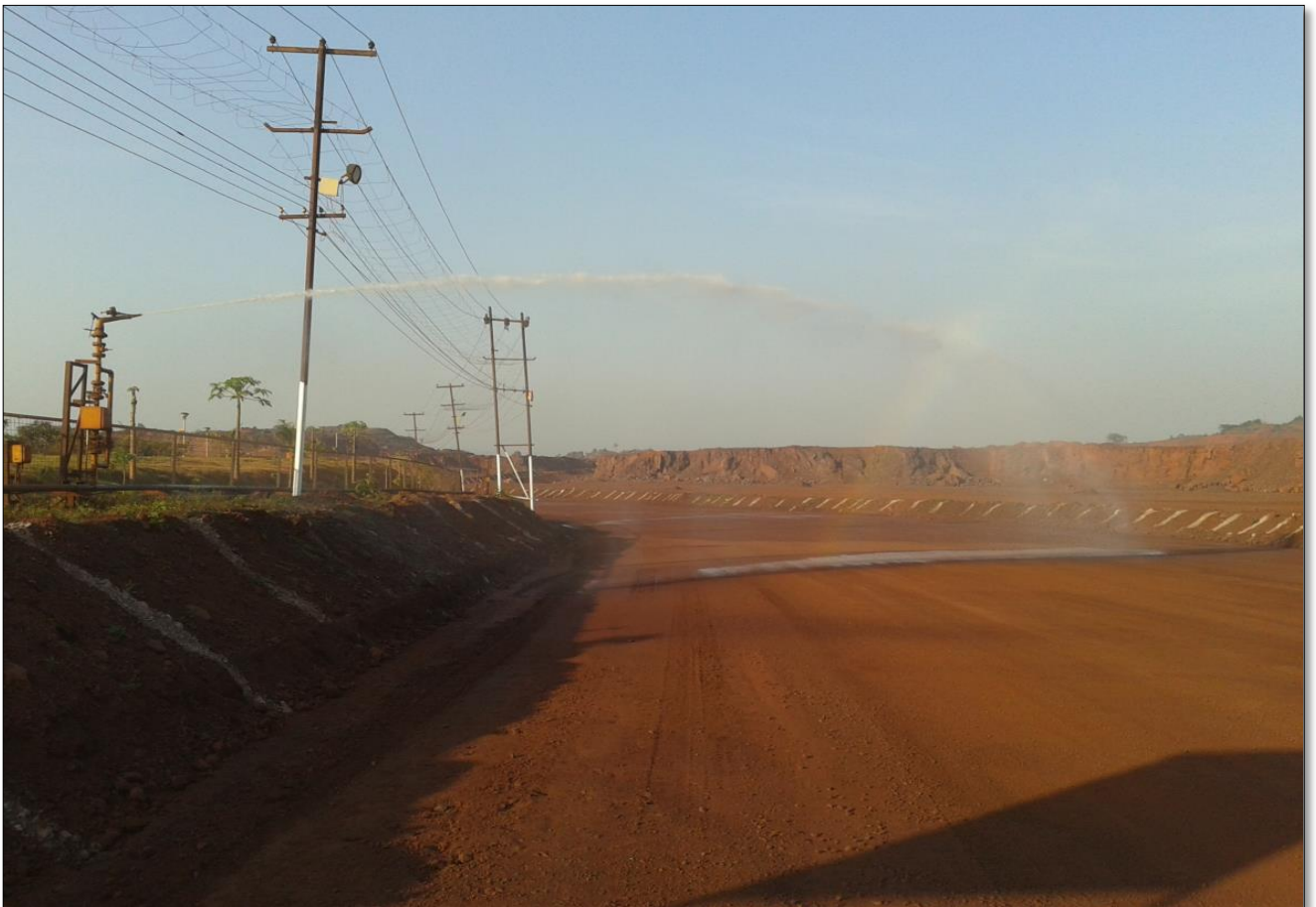
Fixed Water Sprinkling
