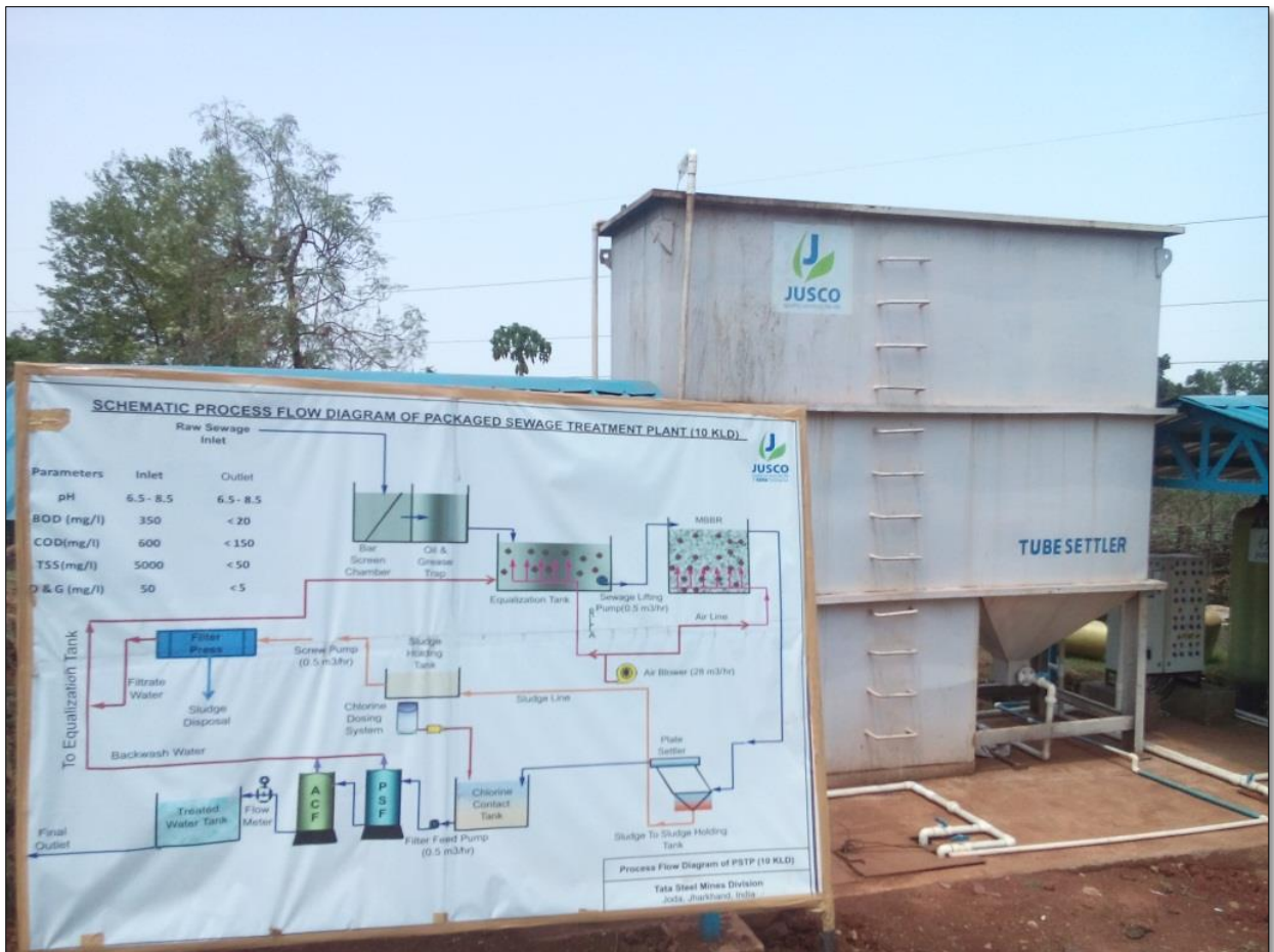
10 KLD STP at Hospital
