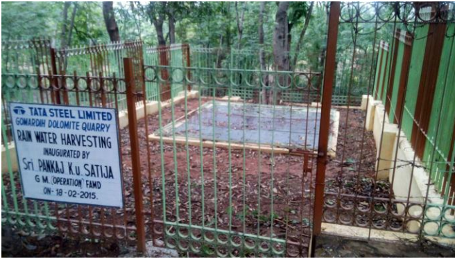
RECHARGE PIT OF ROOF TOP RAIN WATER HARVESTING STRUCTURE OF GUEST HOUSE OF GOMARDIH
