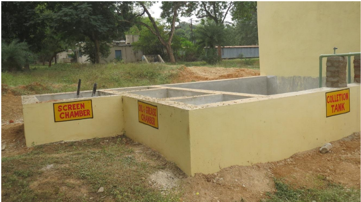
Screen Chamber & Collection Tank
