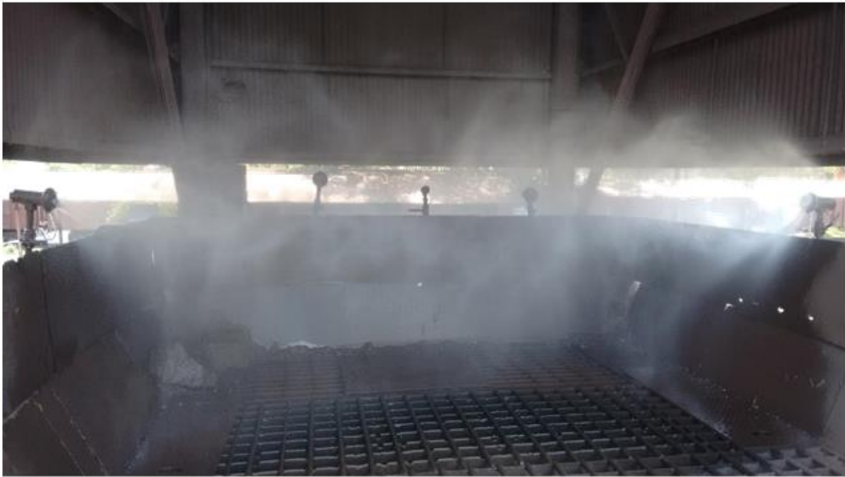
Dry Fogging System for Fugitive dust suppression
