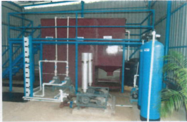
10KLD Effluent Treatment Plant (ETP) at Hospital
