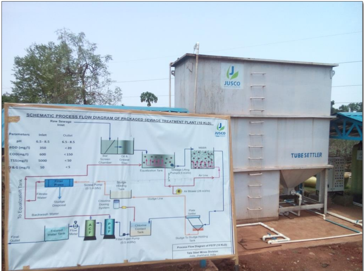
10 KLD STP at Hospital
