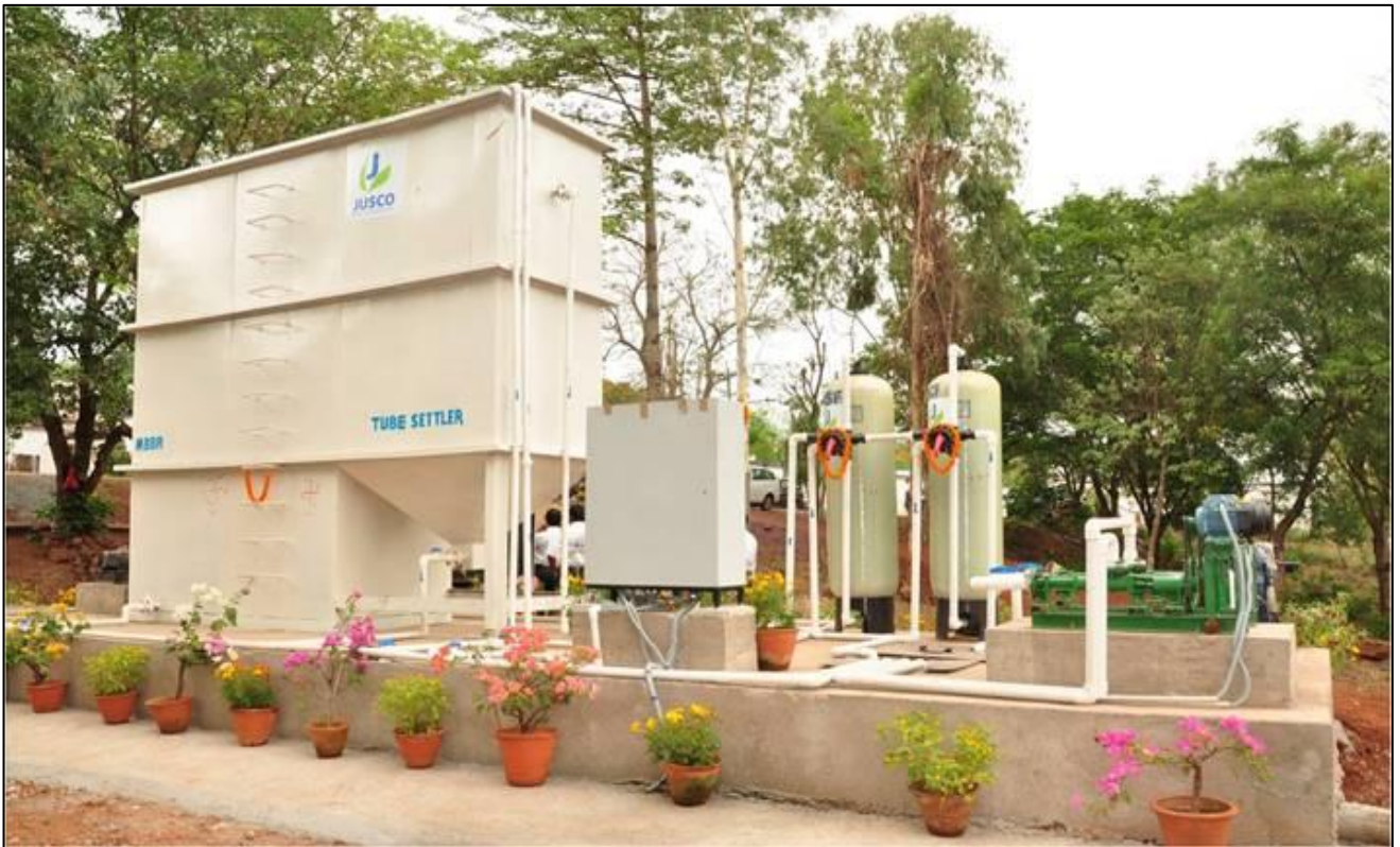
Sewage Treatment Plant
