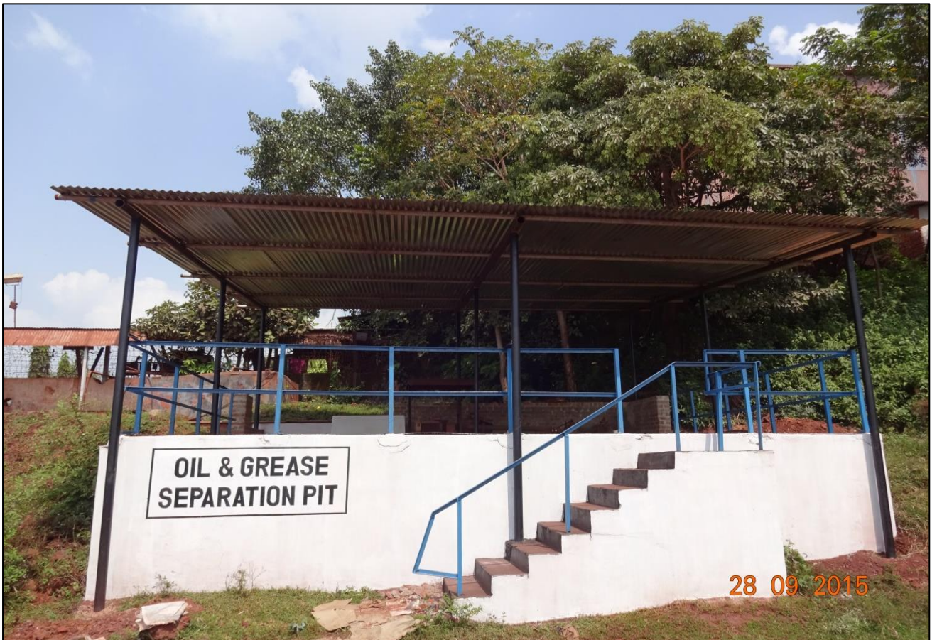
Oil & Grease Separation Pit
