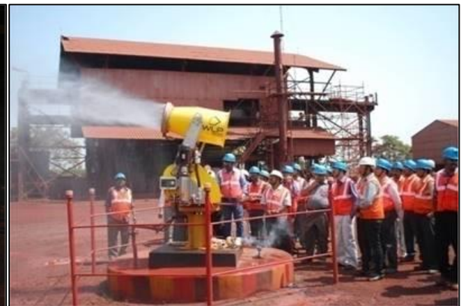
Water Mist System in Plant
