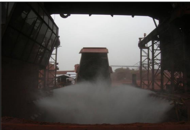
Water Jet System at Unloading Point
