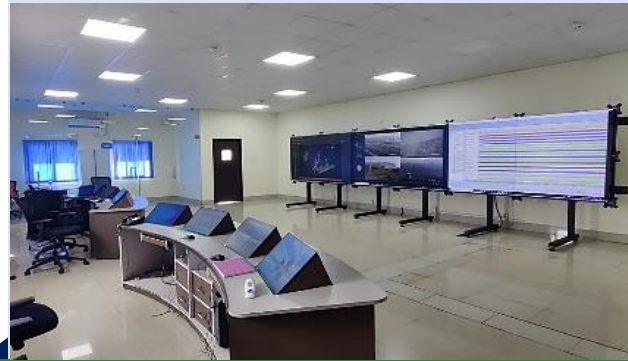
Integrated Command Center to monitor
