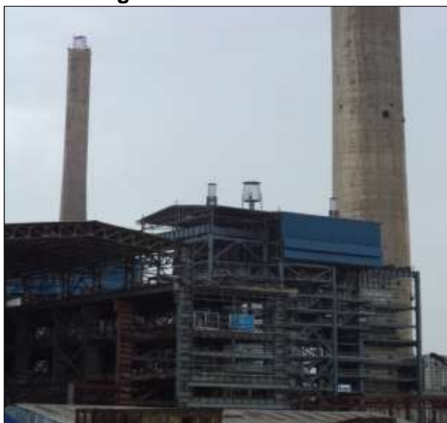
Captive Power Plant
