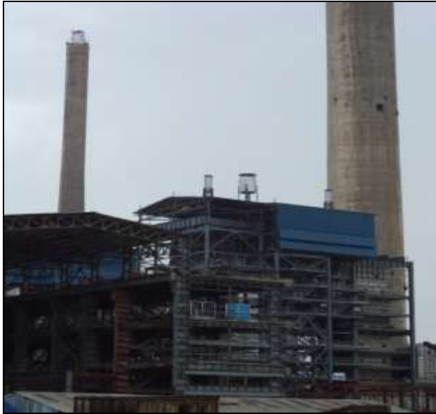
Captive Power Plant
