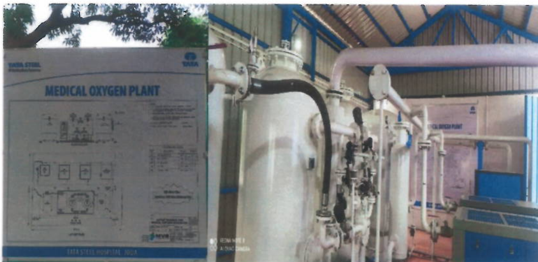
50 Nm 3 / Hr. Medical Oxygen Plant at Tata Steel Hospital, Joda (Sept 2021)
