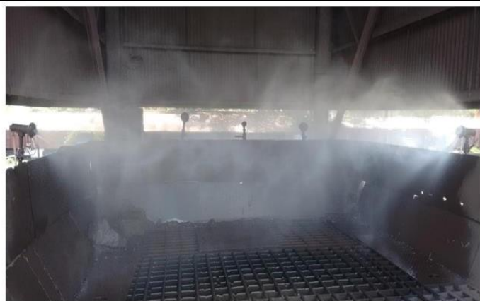
Dry Fogging System for Fugitive dust suppression
