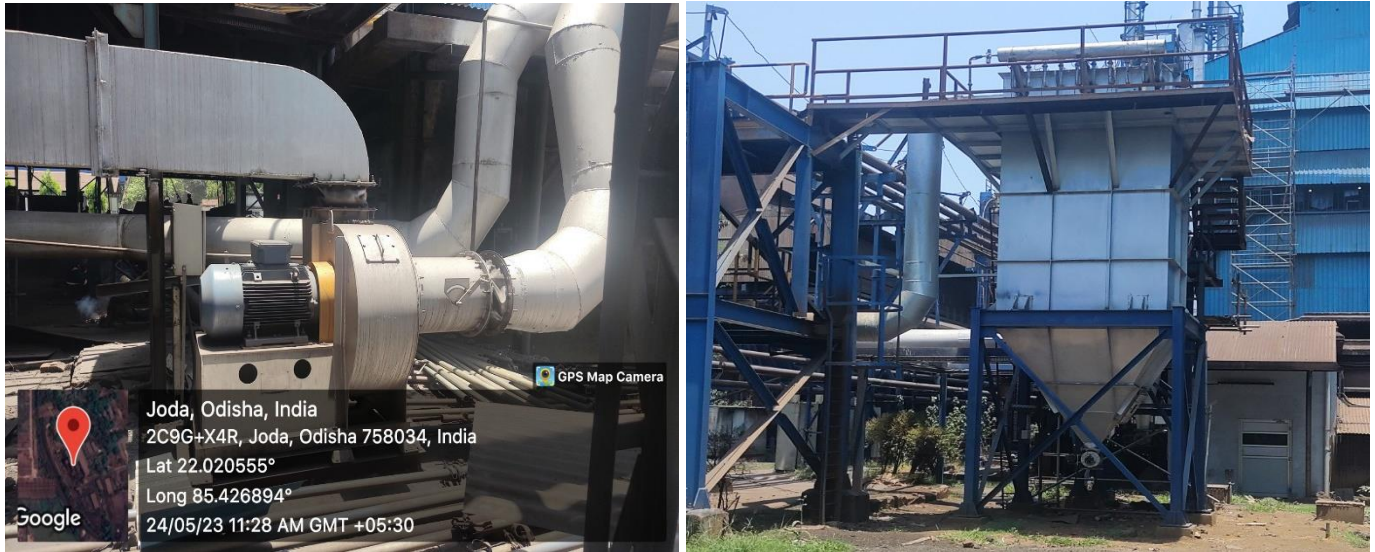
Fume extraction system with bag filter for Tap Hole Emission
