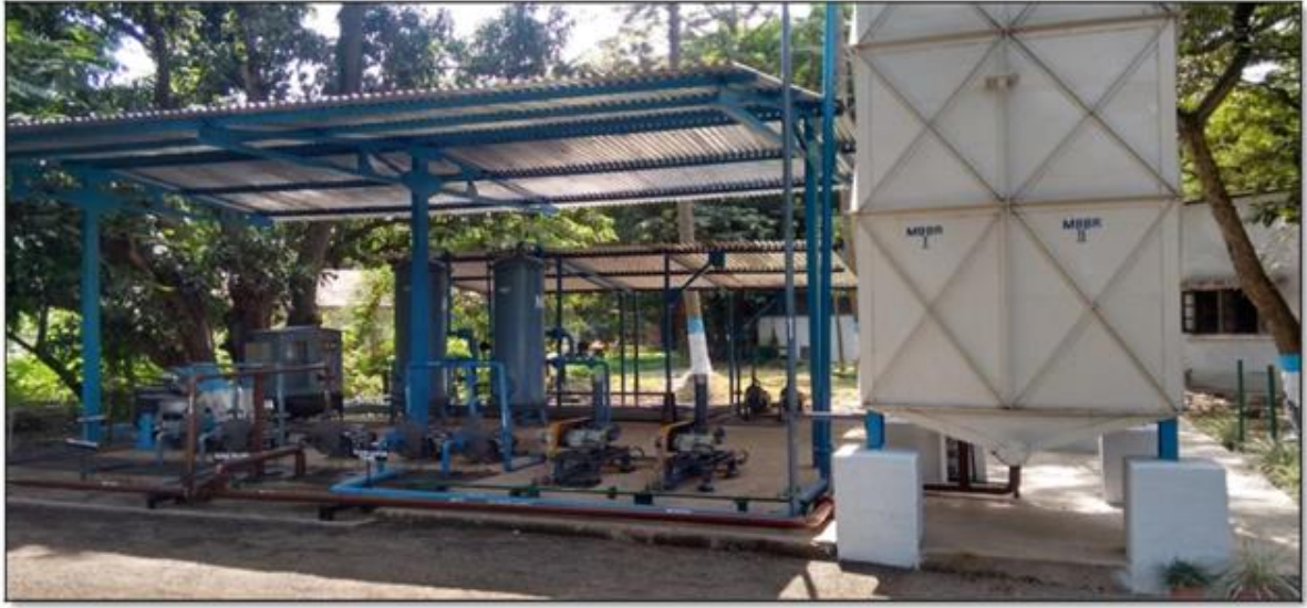
Sewage Treatment Plant Installed at FAP, Joda
