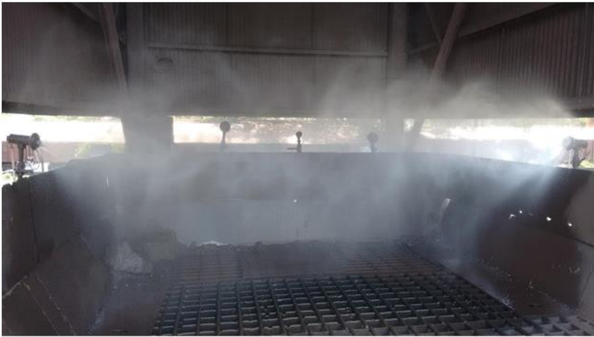
Dry Fogging System for Fugitive dust suppression
