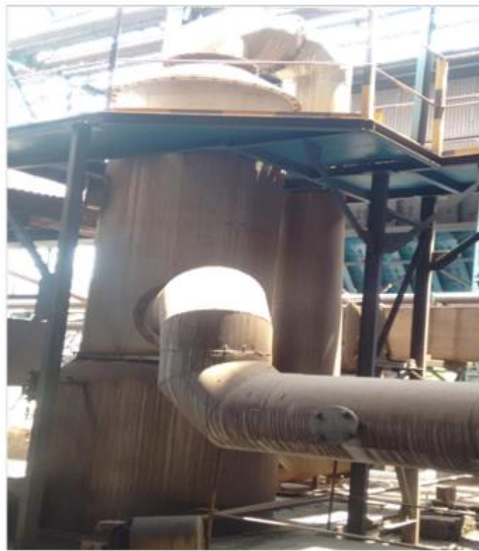
Fume Extraction System For existing Plant
