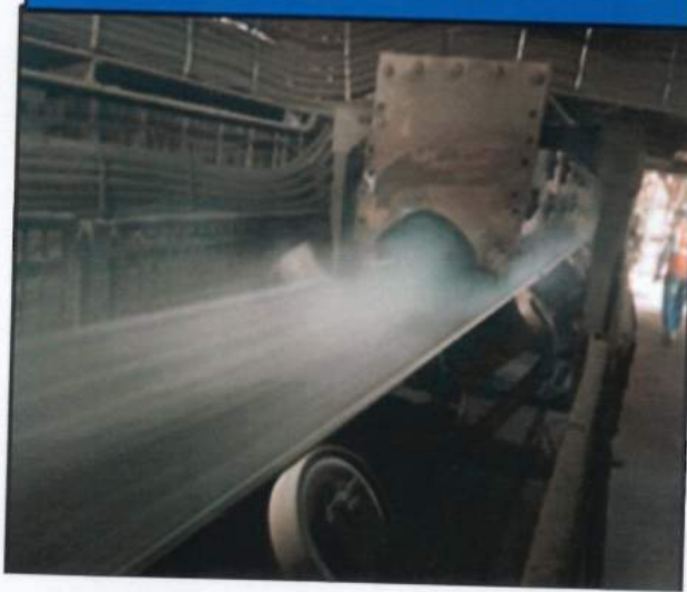
Dry fog system in plants
