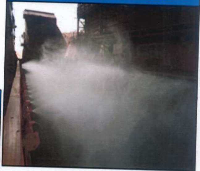
Water Jet system at Primary Crusher
