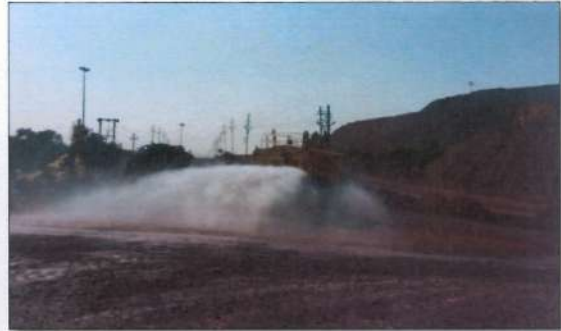
Mobile Water Sprinkler
