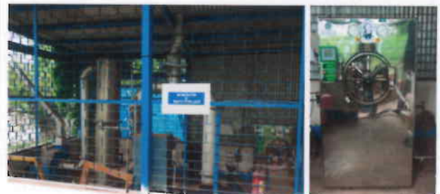
Double chambered incinerator & autoclave at Hospital
