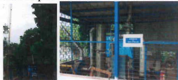
Double chambered incinerator with 60m chimney
