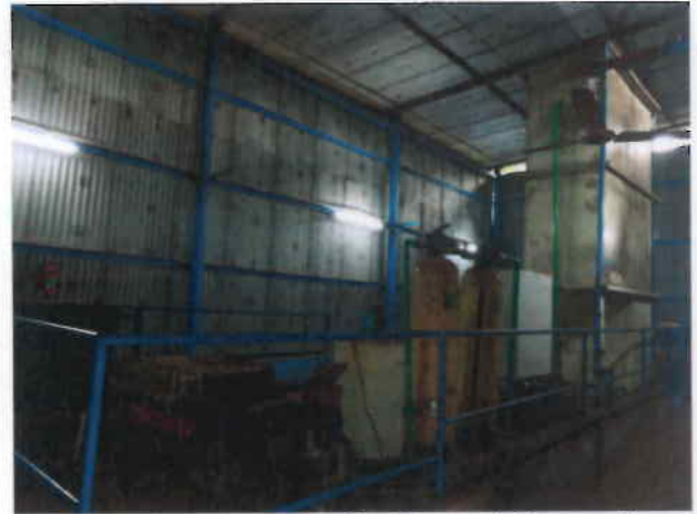
10 KLD STP connected to Hospital, Noamundi
