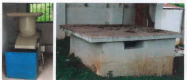
Plastic shredder, ash disposal pit at Hospital
