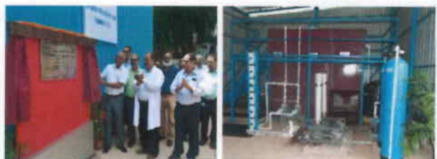
10 KLD ETP at TATA Steel Hospital, Noamundi
