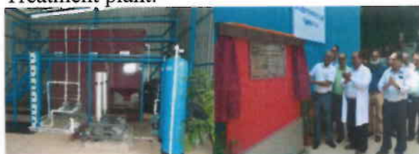
10 KLD ETP at TATA Steel Hospital, Noamundi
