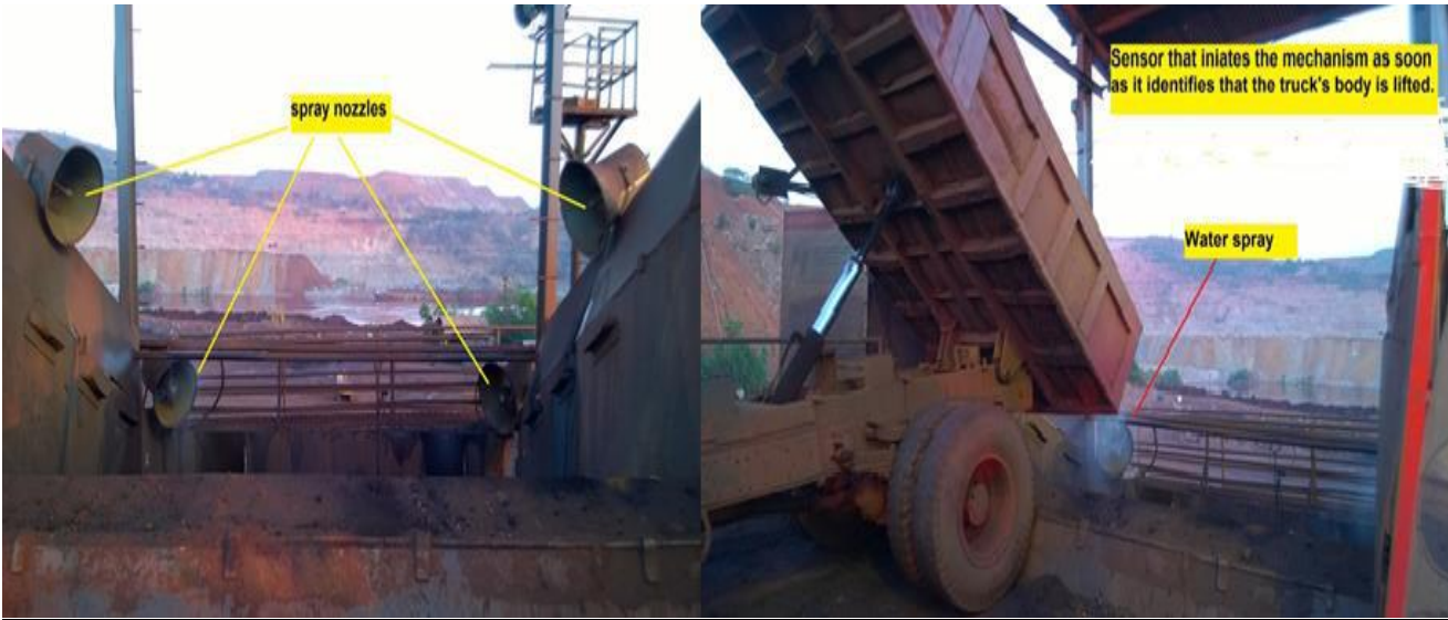
Dust Suppression System at Hopper
