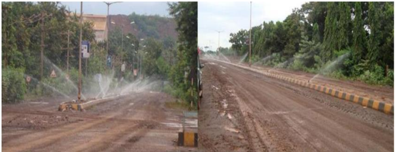
Stationary Water Sprinkler
