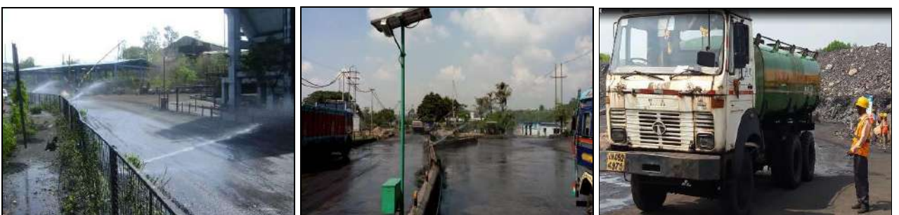
Use of fixed & mobile water sprinklers
