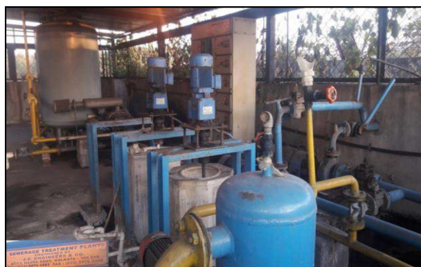
Sewage Treatment Plant (0.24 MLD) at West Bokaro
