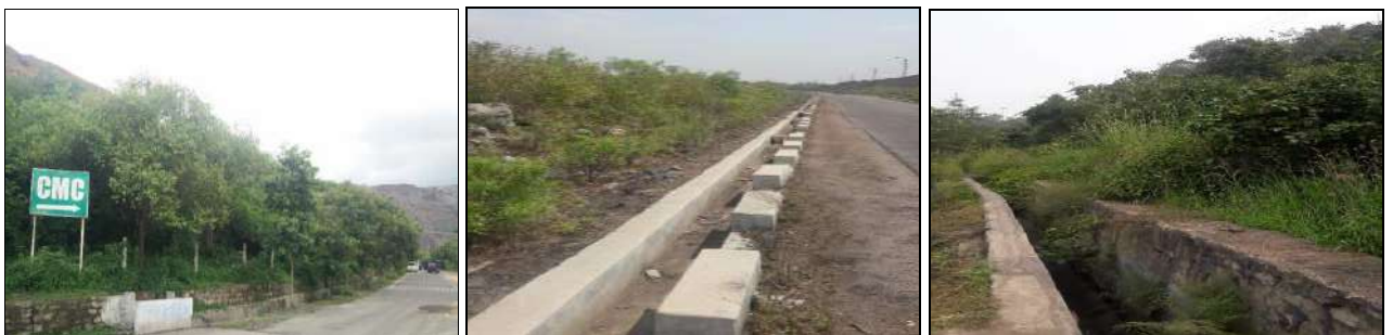
Garland drain in the area
