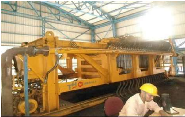
Mechanical tailings de-watering system
