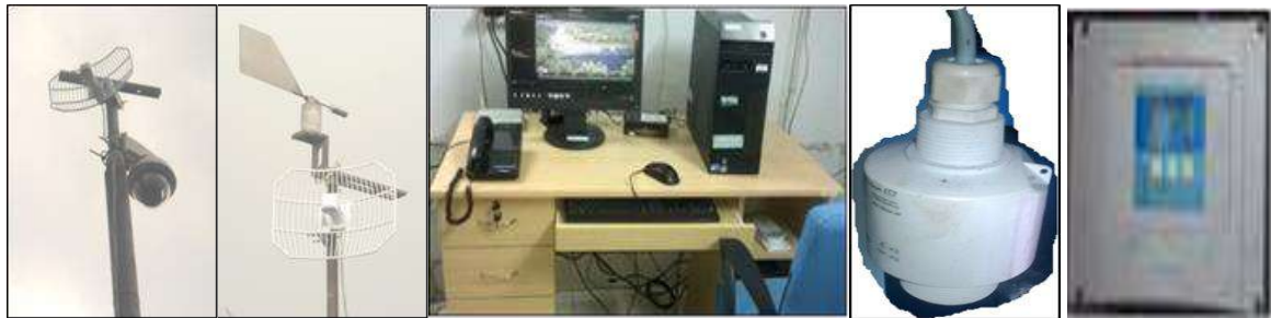
Online Effluent Monitoring System installed at site (Power Plant)
