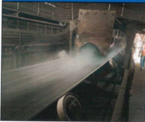
Dry fog system in plants
