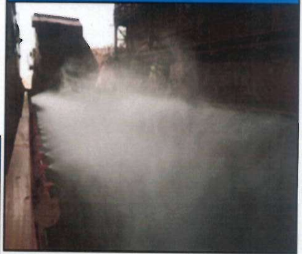
Water Jet system at Primary Crusher
