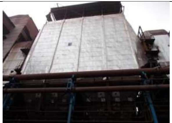
Sinter Plant 2 Waste Gas ESP
