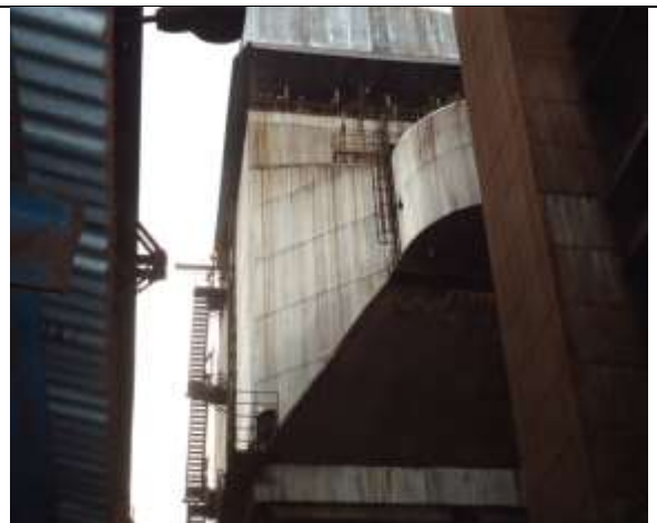
Sinter Plant 2 New Waste Gas ESP
