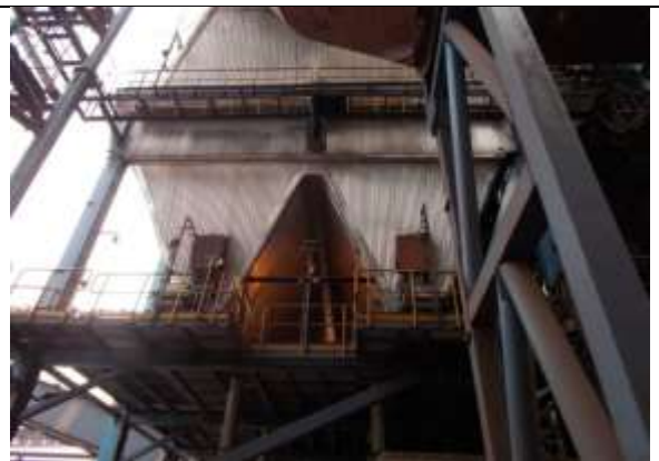
Sinter Plant 3 Refurbished ESP
