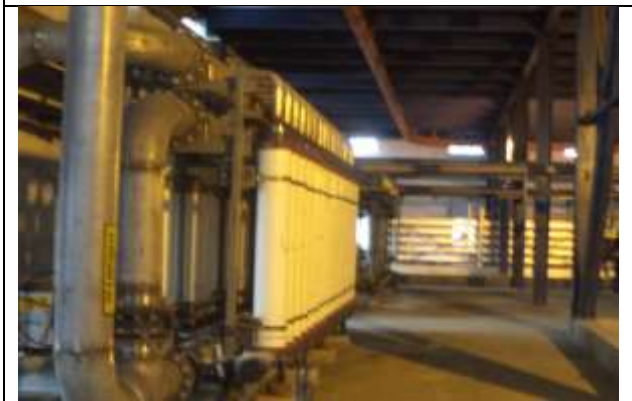
Reverse Osmosis Plant
