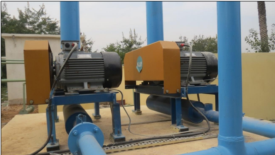
Intake Pump station
