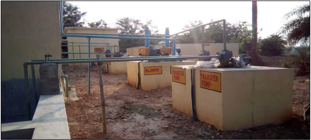
Screen Chamber & Collection Tank
