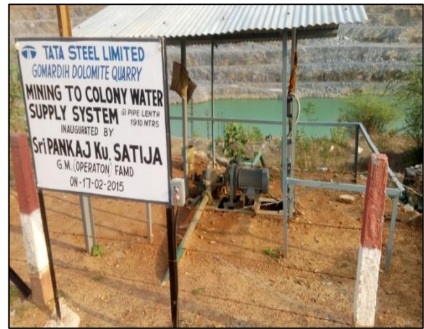
ARRANGEMENTS FOR PUMPING AND TREATMENT OF ACCUMULATED RAIN WATER OF THE QUARRY
